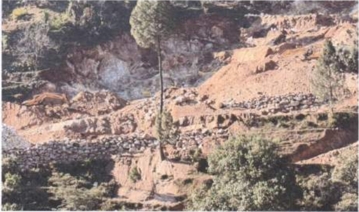
Earth Moving Equipment at Work in front of Road at GPS Coordinates 79° 47' 51.39" E 29° 52' 7.848" N
