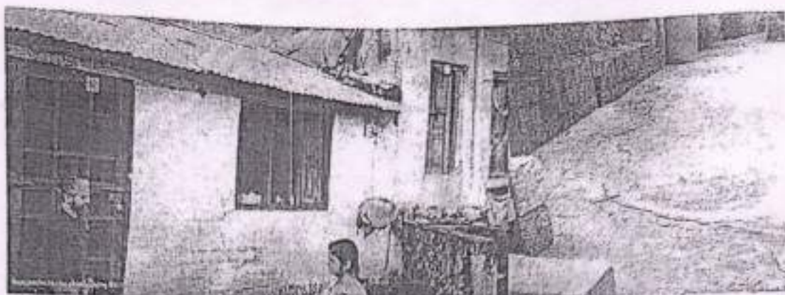
Fig. 3: Field photograph showing cracks in House-1 of Kanda Kaniyal Village.
